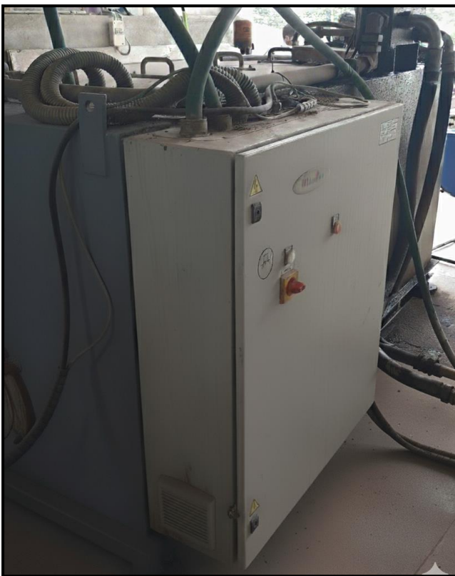
Hydraulic Power Unit
